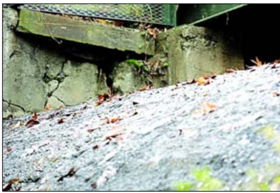
A section of Lake Neepaulin dam structure shows the wear of age.
